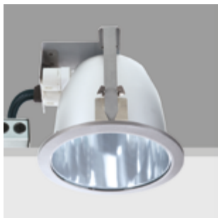
Outdated installation with recessed downlights
