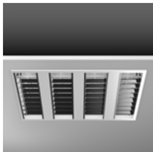
Outdated installation with mirror louvre luminaire
