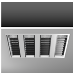
Outdated installation with mirror louvre luminaire
