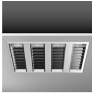
Outdated installation with mirror louvre luminaire
