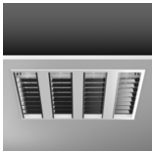
Outdated installation with mirror louvre luminaire
